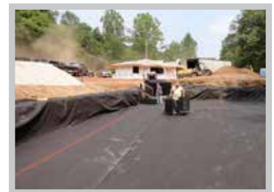
Fig. 7 Use a string line and marking paint to square the system footprint.
