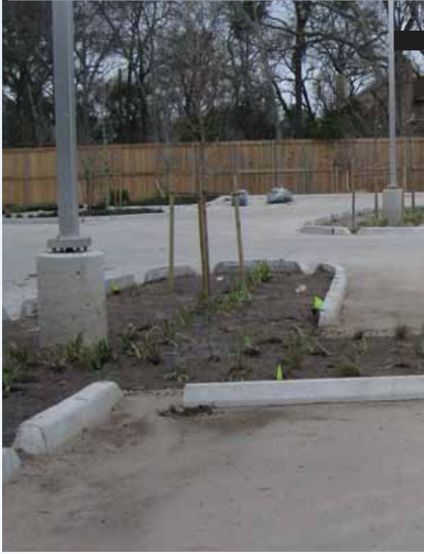
BEFORE: Slow Flow Engineered Media Clogged Bioretention System
